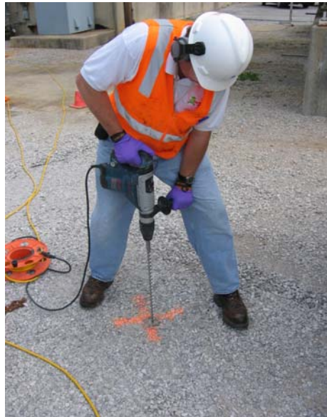
FIGURE 2. Using a compression drill to create the installation hole for the GORE™ Modules.
